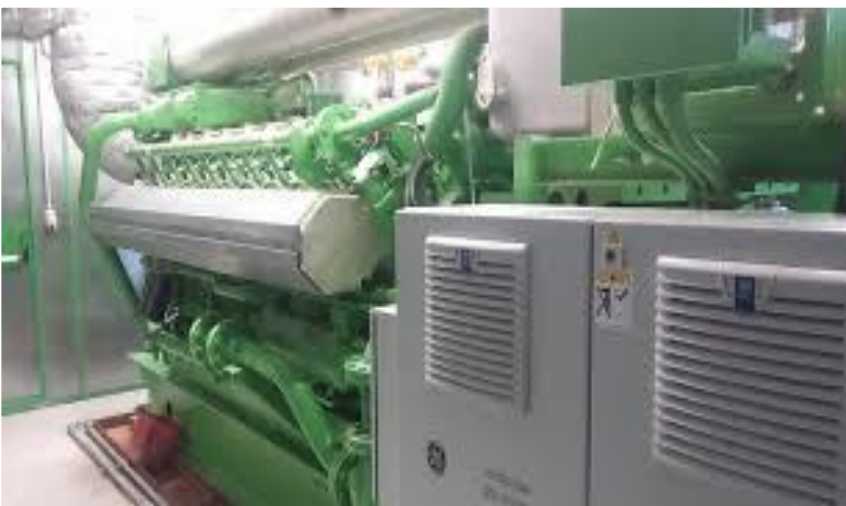
COMB. HEAT & POWER UNIT
