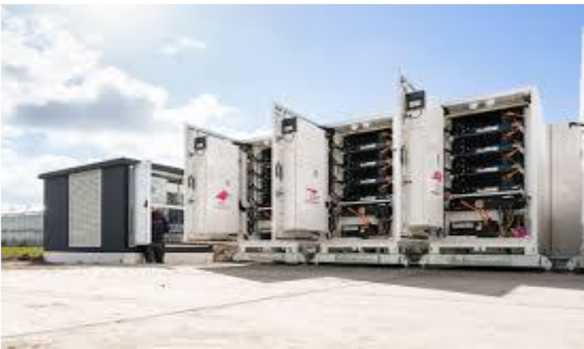
DYNAMIC BATTERY SYSTEMS
