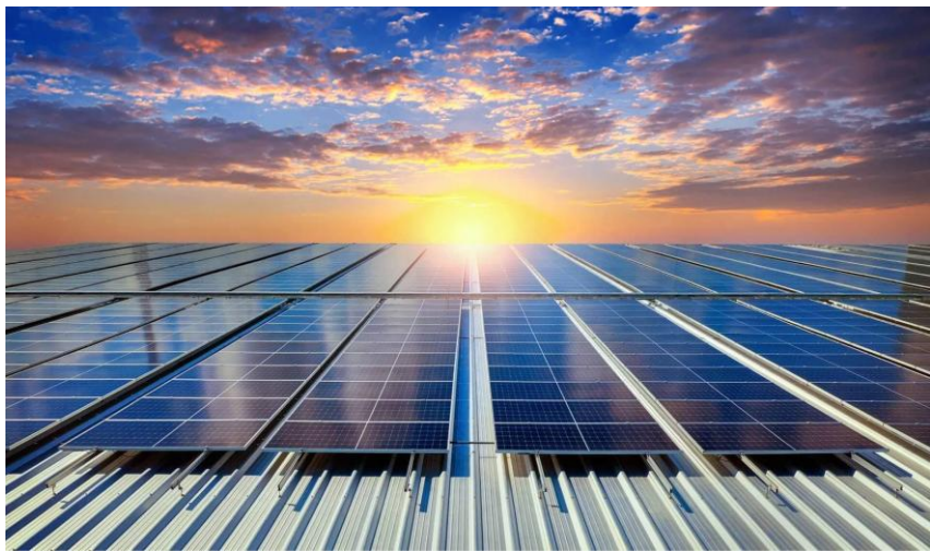
INTEGRATED SOLAR PV
